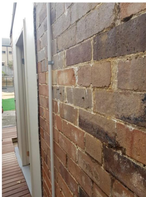
Plate 8: Northwest wall of property showing junction between brick and fibre-cement sheeting extension.
