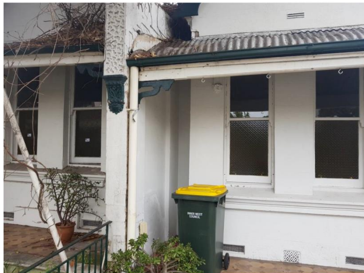
Plate 3: Detail of damage to bullnose verandah.
